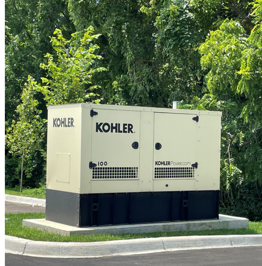
Building Generator for Life Safety Systems
